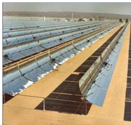
Fig. 2 Parabolic Trough arrays
