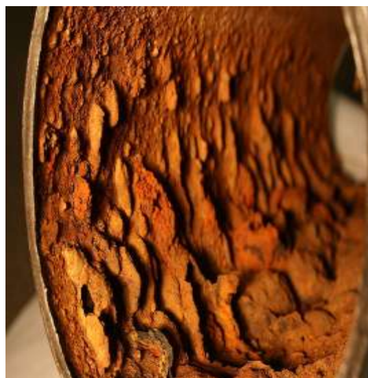
Figure 1.8: MIC corrosion inside a fire sprinkler systems
