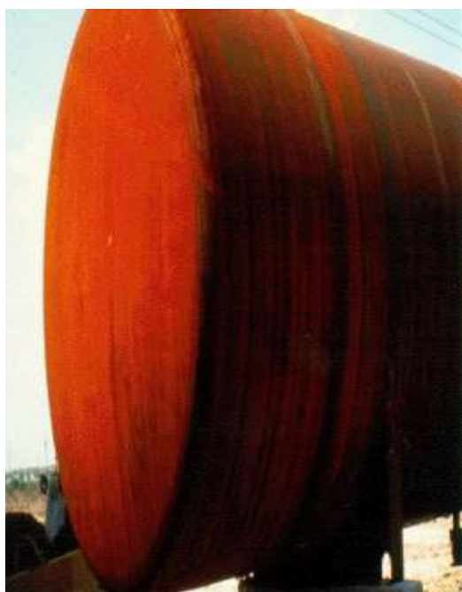
Figure 1.2: Uniform corrosion on a storage tank
