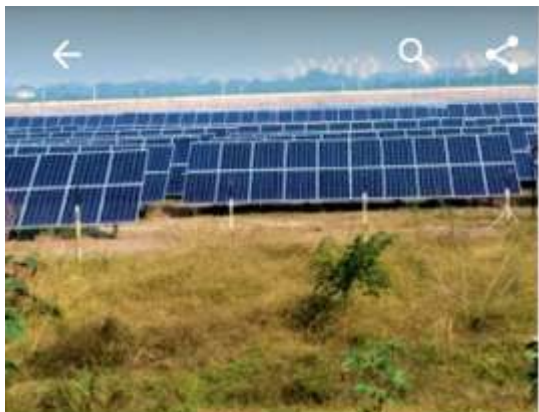
10MW SOLAR POWER PLANT, VISAKHAPATNAM PORT TRUST
