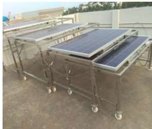
ROOF TOP SOLAR POWER PLANT
