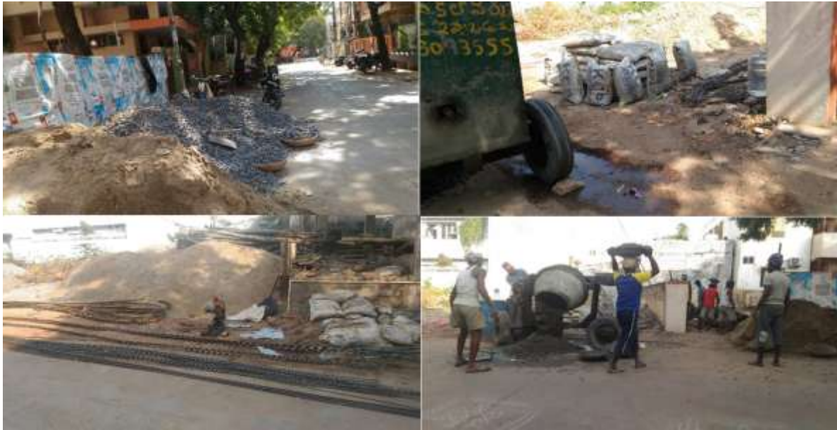
Figure 7: Stacking of construction materials on the street (top & bottom left), Concrete mixing on street (bottom right)
