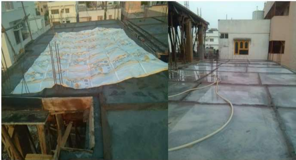
Figure 5: Covering fresh concrete with Tarp (left), Water curing the completed slabs using curing pond method (right)
