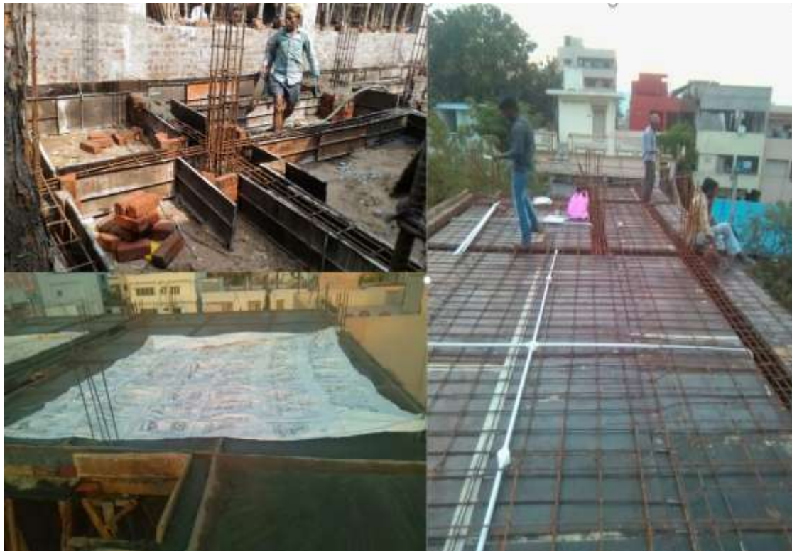
Figure 9: Misalignment of beam formwork (top left), unsafe work conditions (right), fresh concrete prone to rain flooding-inadequate cover (bottom left)
