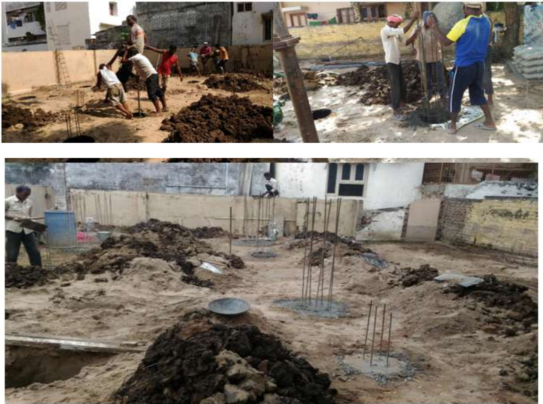
Figure 1: Workers drilling augurs for concrete piles (top left), placing steel reinforcement into the pile shaft and concreting (top right), foundation steel extended up to tie with column steel(bottom)
