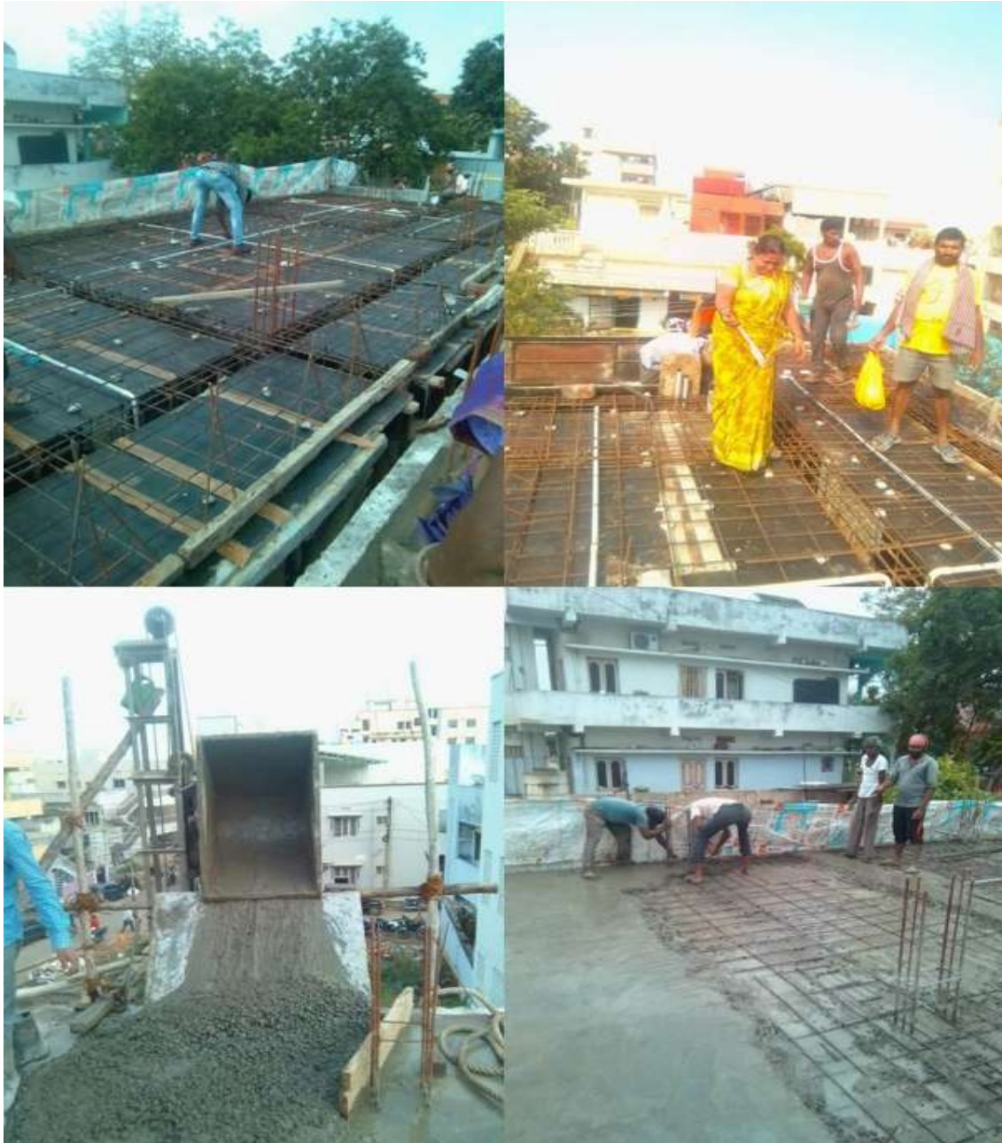
Figure 4: Worker tying slab reinforcement on stop of formwork deck (top left), Engineer inspecting reinforcement details (top right), slab concrete pour from chute (bottom left), workers doing concrete finish (bottom right)
