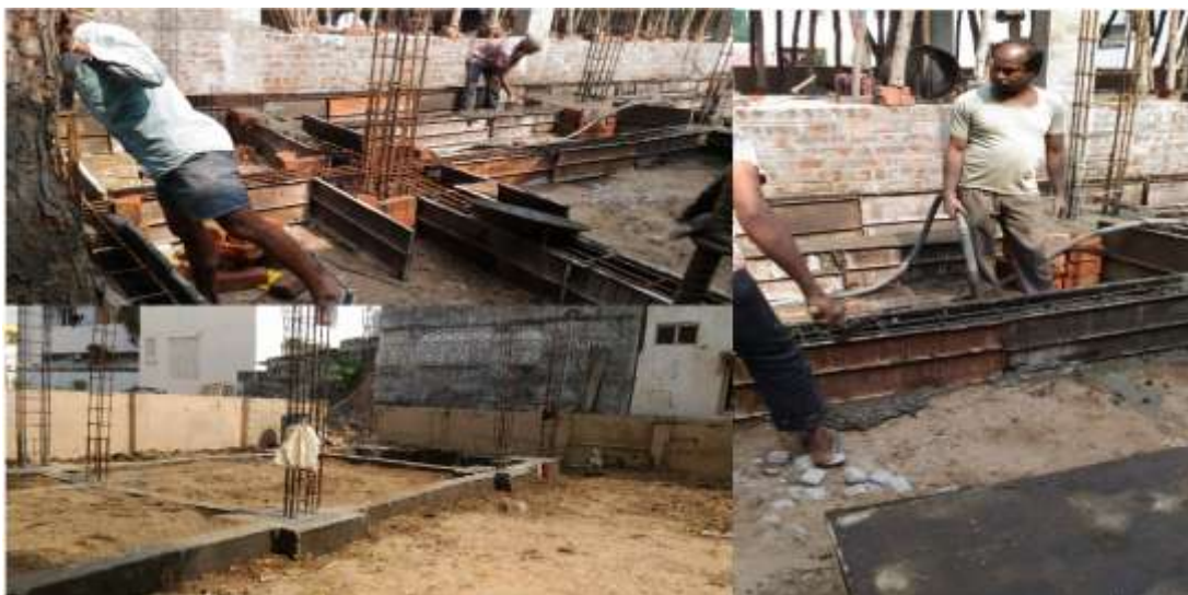
Figure 2: formwork for plinth beams (top left), plinth beams being concreted & compacted (right), completed plinth beams with column steel in place (bottom left)
