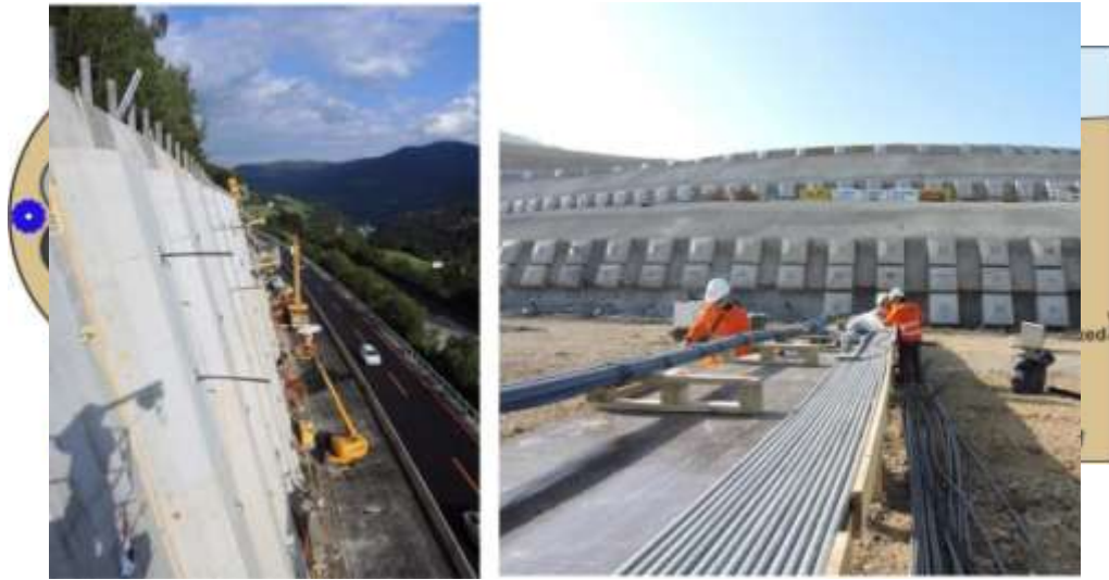
Figure 6. Slope stabilization using ground anchors for retaining walls at highway (left) and at a refinery(right) Figure 7. Schematic representation of single borehole multiple anchors with two sensing fibres along the tendons of
