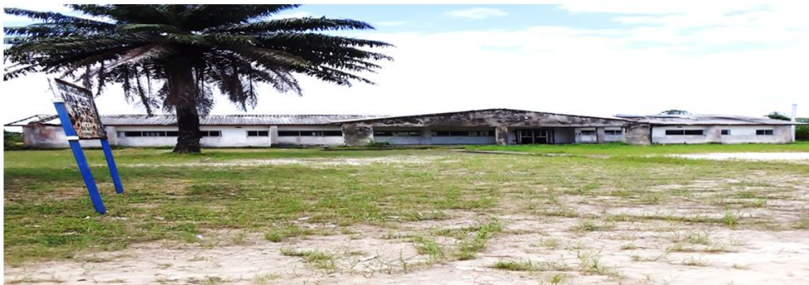
Plate 1: Dilapidated and Abandoned PHC Facility in Oloma Community in Bonny LGA Source: Researcher's Field Survey, 2020
