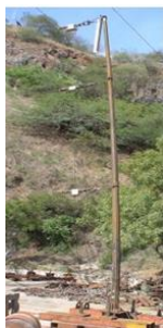
Figure Tubular steel pole
