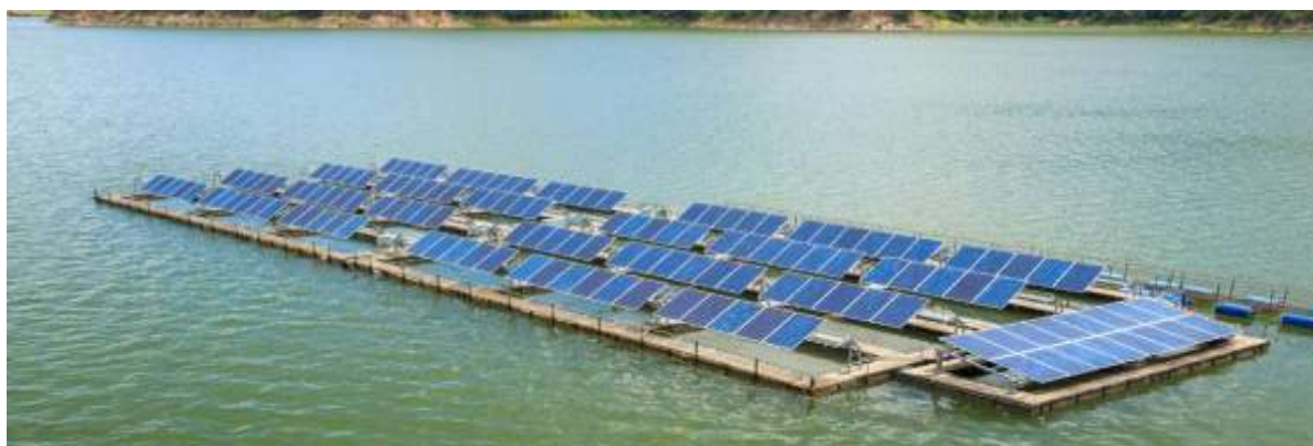
Floating Solar Power Plant
