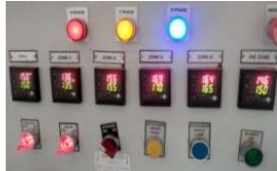
Figure 17. Twin Screw Extruder Control Panel
