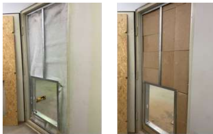
a) Insertion of Recycled-PET fiber insulation in the LSF wall b) Insertion of vermiculite boards in the LSF wall
