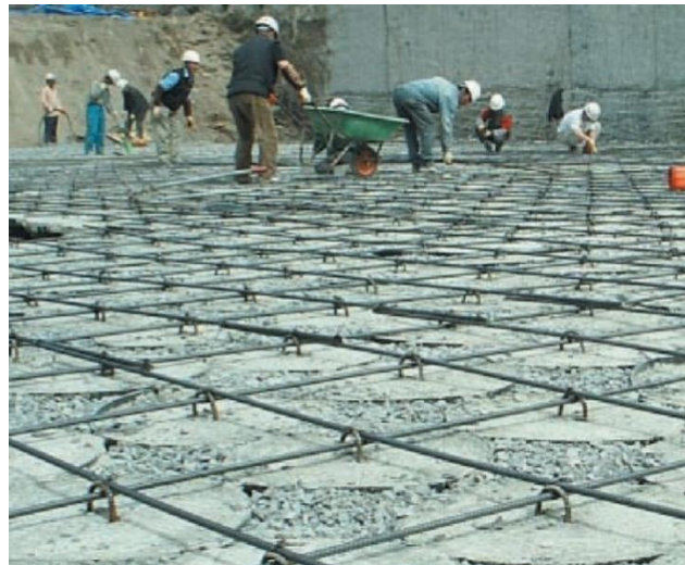
STEEL MESH INSTALLATION AND CONCRETE PLACEMENT TO FINALIZE THE TOP-BASE FOUNDATION STRUCTURE
