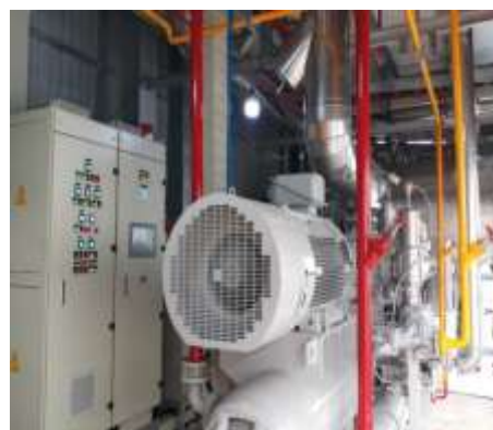
Figure 1. The industrial refrigeration system
