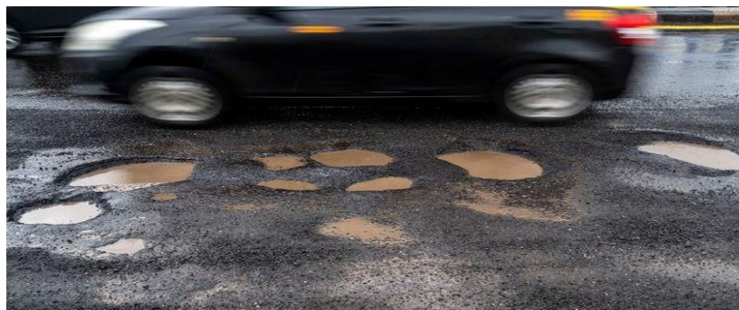
Plate 1: Cracking and Potholes
