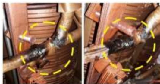
Figure 7: LV winding failure in the Y connection.
