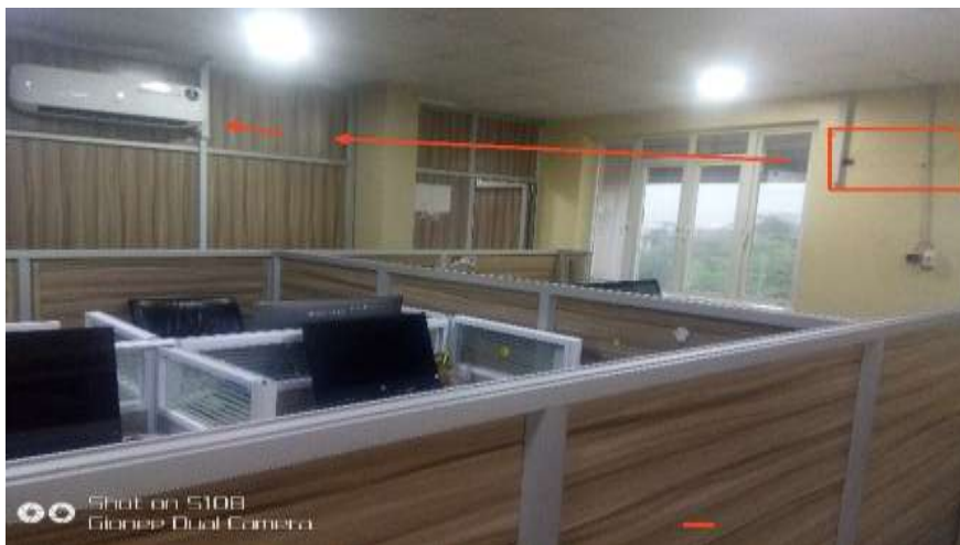
Figure 18: Showing the new position of the second AC from the red box to the current position
