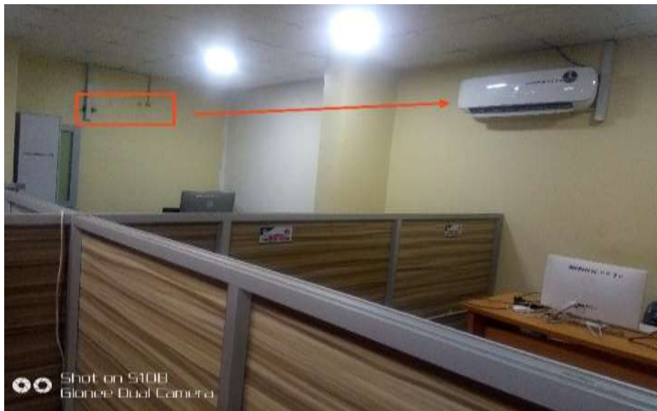
Fig.17: Showing the new position of the two ACs from the red box to the current position
