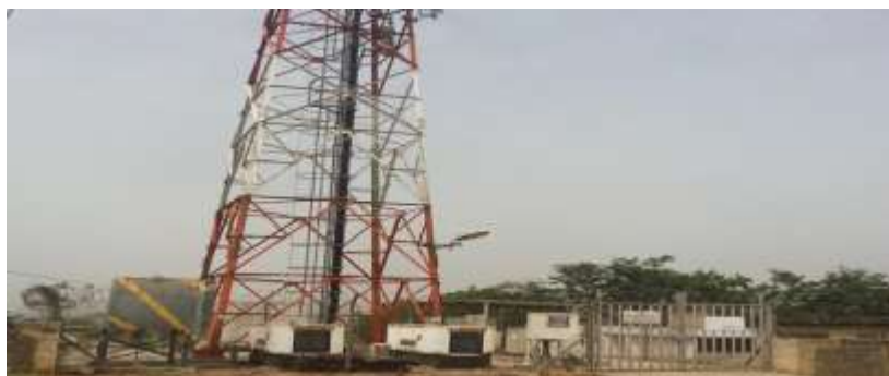
Figure 3. Typical outdoor cellular base station
