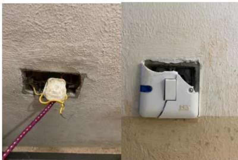
Pictures of showing bad electrical connection and a bad fitting – Akindeko Hostel Source: Author (2023)
