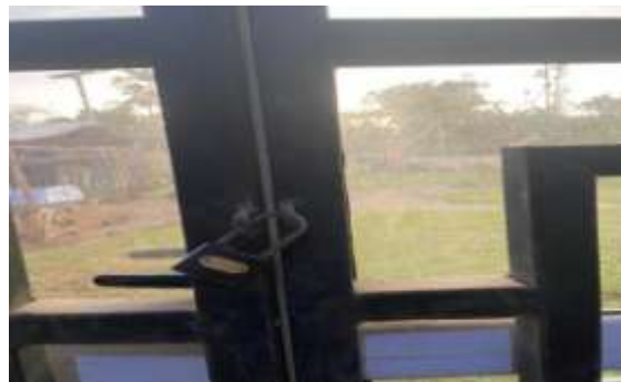
Picture showing a locked emergency exit at the P. Adeniyi Hostel Source: Author (2023)
