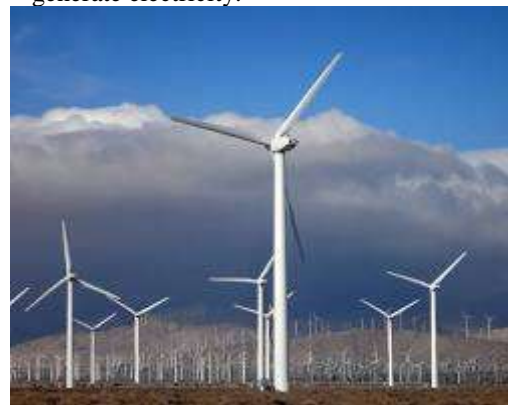
Wind power plant
