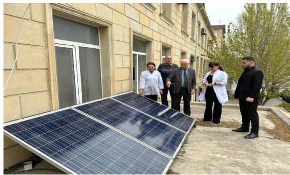
Figure 2. General view of the SPP with a power of 750 W and consisting of 3 SPs installed on the facade at the entrance to the Institute of Radiation Problems
