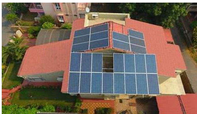
Fig-3: It shows a rooftop based Photovoltaic (PV) System.
